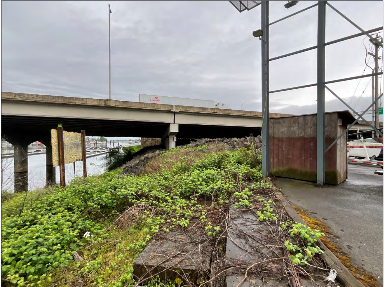
Figure 10. View of Columbia River Levee, north side, view facing east (WillametteCRA May 4, 2023).
