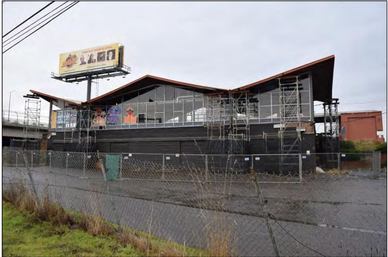
Figure 6. View of 1415 North Pier 99 Street prior to demolition of second story and roof, facing north (WillametteCRA January 16, 2023).
