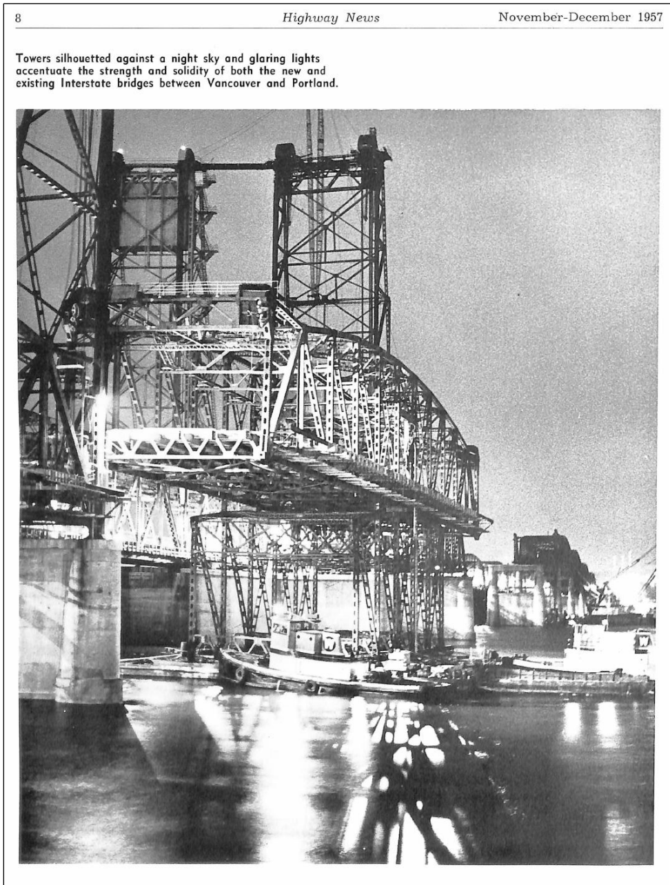
Figure 12. Photograph of the lift span being raised into place (Washington State Highway Commission, Highway News , November-December 1957).
