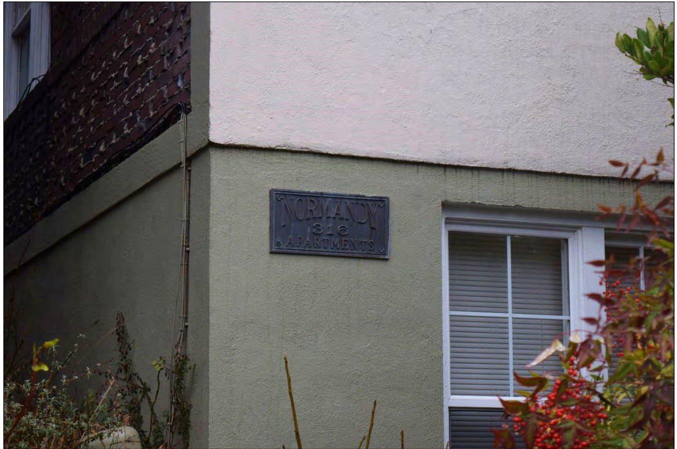
Figure 8. Detail of the south elevation of the Normandy Apartments showing a replaced window, view facing north (WillametteCRA January 16, 2023).
