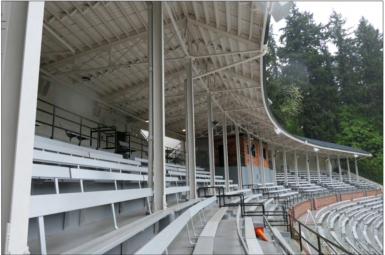
Figure 13. Kiggins Bowl stadium, detail of metal truss substructure. View facing northwest (WillametteCRA May 6, 2023).
