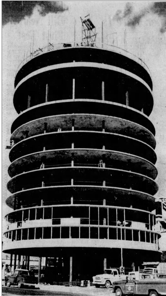
Figure 18. Construction photo showing lift slab construction method ( The Columbian [Vancouver, WA], April 5, 1965, 1).
