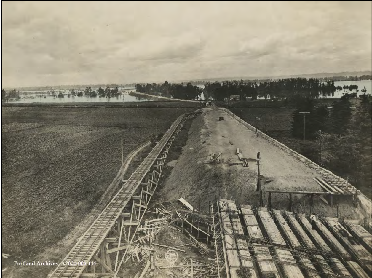
Figure 19. Union Avenue (present-day NE Martin Luther King Boulevard) under construction in 1916. View looking north-northwest. The partially constructed viaduct over the Oregon and Washington Navigation Company tracks is in the foreground while the line's shoefly is seen on the left (City of Portland Archives, A2001-008.144).
