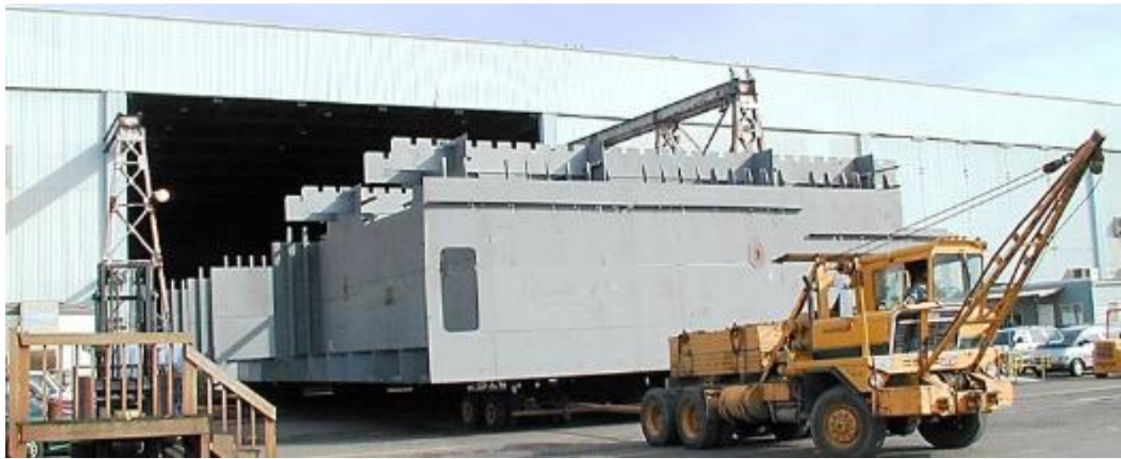
Shown above and below is a modular segment of the Power Barge fabricated by TMF. Segments were pre-fabricated in the shop before being assembled in Thompson's yard. The final assembly was 105' W x 30' H x 284' L
