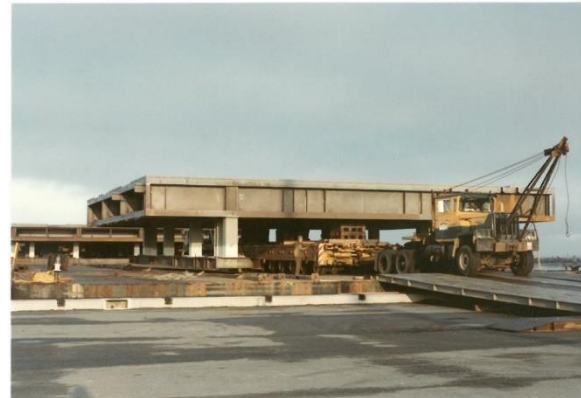
The platforms (seen left) were delivered by barge to Alaska where high capacity trucks and dollies (shown above) off loaded the structures for delivery to the jobsite.
