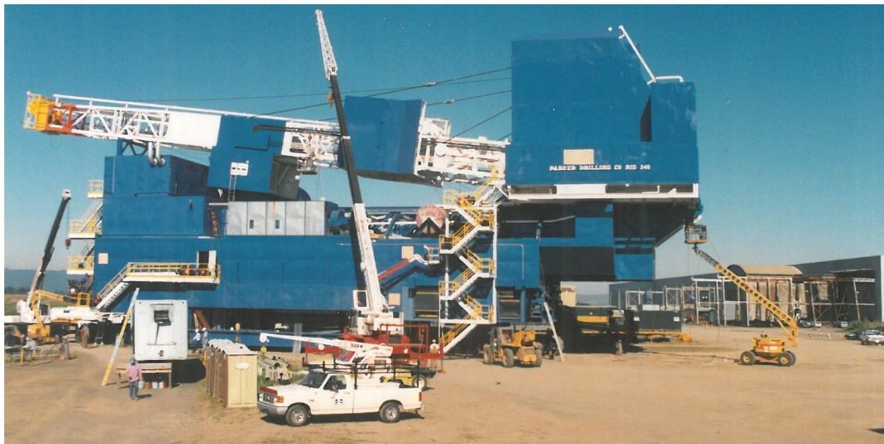
Parker Drilling Rig 245 being ‘rigged up’ at Thompson Metal Fab’s yard. This yard space is immediately adjacent to the manufacturing facility and to the roll-on/roll-off barge slip. The ability to offer turnkey projects and delivery via water has given Thompson Metal Fab an advantage in the marketplace.
