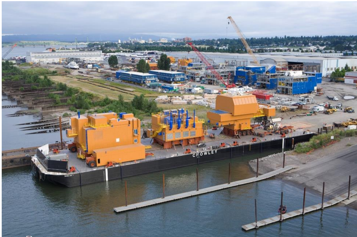
Doyon Drilling Rig 25 shown on the barge in the foreground. Due to the size of the rig and its six mega-modules, two barges were required for delivery to Alaska's North Slope. The background shows the remaining modules for Rig 25, in addition to Parker Drilling's AADU Rigs (Rig 272 and Rig 273)
